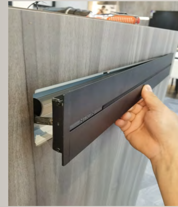
5 Insert and tighten the Electric cables to the "Live", "Earth", "Neutral" part of the end terminal as per indicated and screw on the end terminal cap
